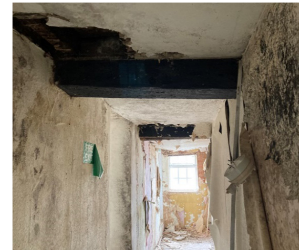
In the foreground, one of two new joists spanning the building front to back inserted to allow the rear access passageway to be cut through the timber frame, the second black painted "beam" is fake.
