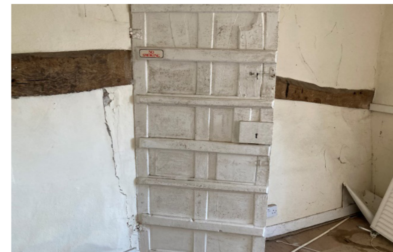
18th century six panelled door into new bedroom, the door is heavily re-enforced on the east side.
