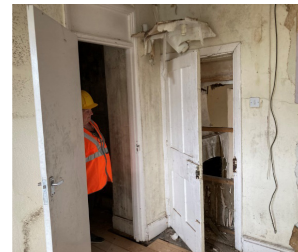
Mid-19th century door to allow access to the assembly room from the easterly bedroom.
