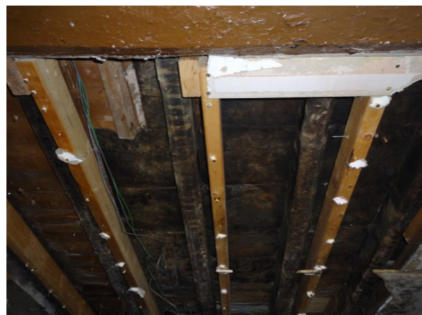
Above - Stepped stop to chamfer on the main beam running east west from the fireplace. Below - soot covered floorboards and chamfered joists running north south with curved ends and stops, evidence of later lathe and plaster and then plaster boards ceiling applied on top of these.
