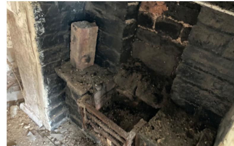
Left - possible frame to skylight in attic. Right - early 18th century fireplace in eastern most bedroom.
