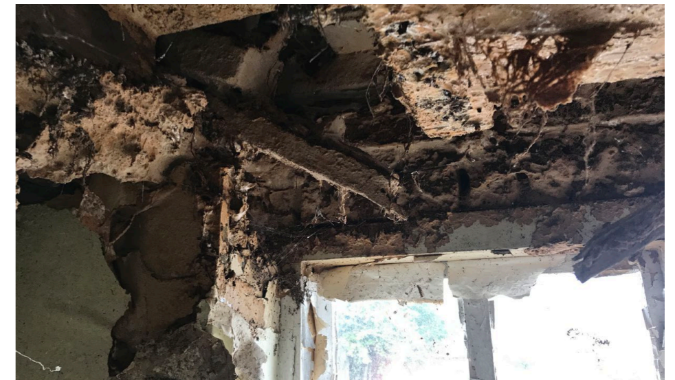
Existing ceiling and timber structure in disrepair
