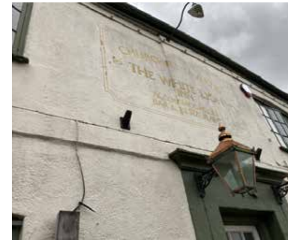
Vertical step in the frontage between the two 17th century phases of build.
