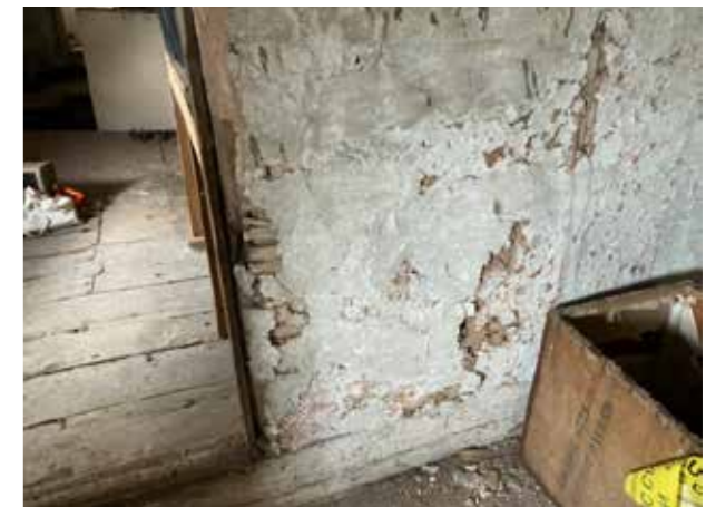
Above - original external timber frame at first floor level keyed to enable render to be applied. Below - split lathe and thick lime render to what was the external wall visible in the attic space.
