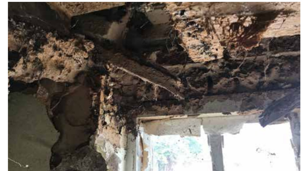
Existing ceiling and timber structure in disrepair
