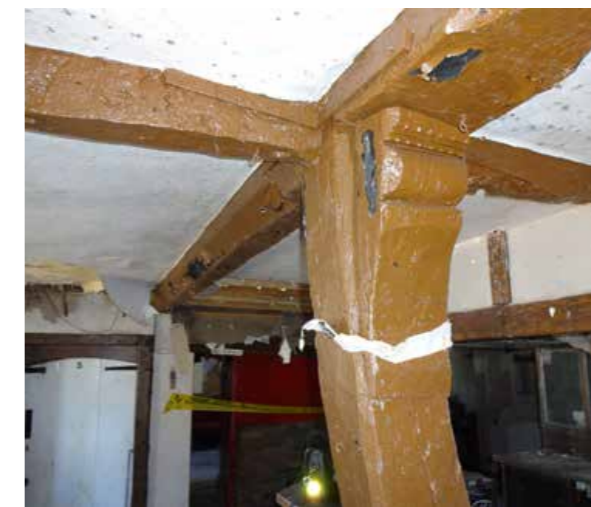
Vertical timber remains of the end wall at ground level with chamfers either side, that in the original phase is much deeper. Mortice holes from the original ground floor end wall visible.
