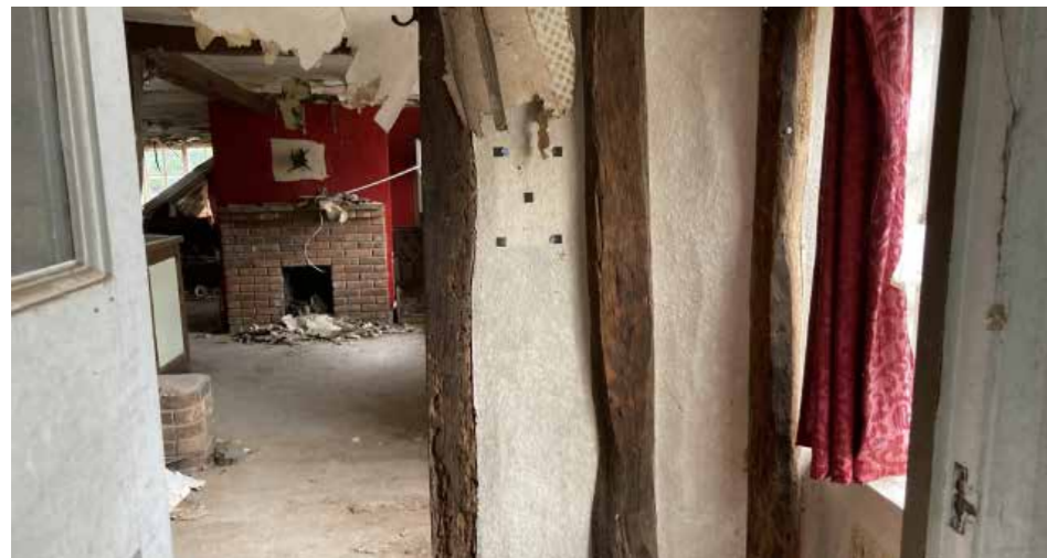
Historic pieces of timber help form a draft screen but do not join into the timber frame and cut across one window.
